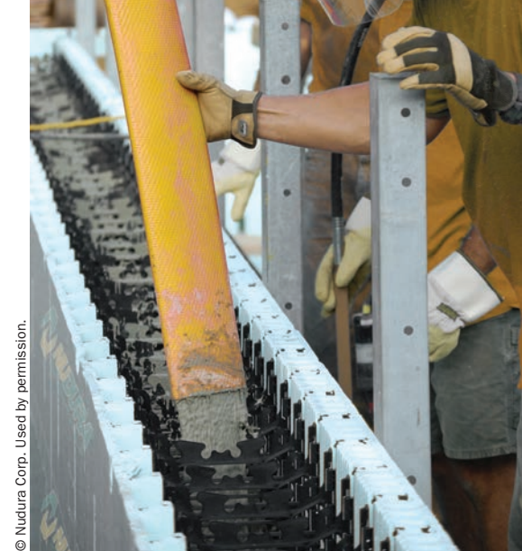
Richardsville was constructed using insulated concrete form (ICF) walls that enhance the building's thermal envelope.
